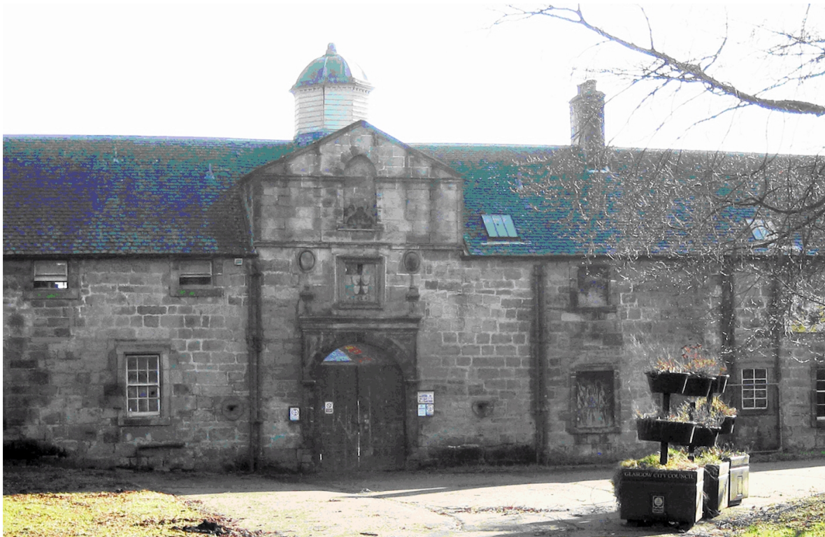
The formal entrance to the Stables courtyard at Pollok House in February 2019, prior to the onset of the restoration. (Bob Powell)
